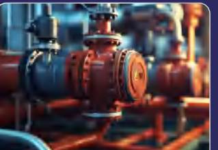
Pumps and general connections
